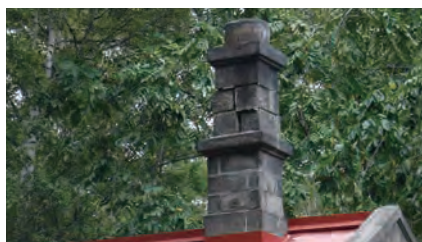
Food Processing Plant of the Model Barn (distorted masonry chimney)
